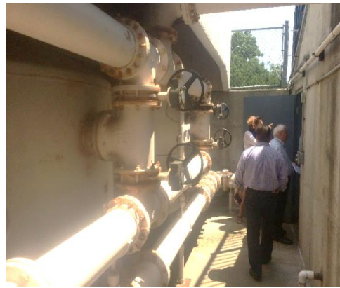
Merriam Aquatic Center Filtration Room
